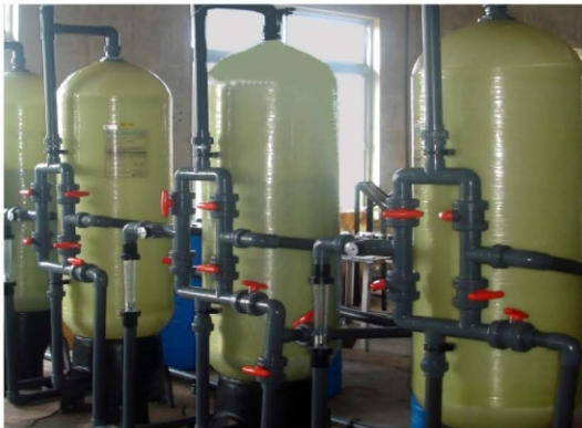
Arsenic Removal Plant for Ground Water Treatment
