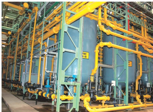
Uranium Recovery Plant at Mining Industry
