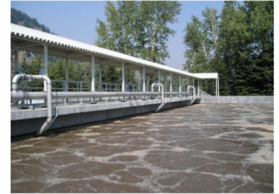
Drinking Water Treatment for Municipality
