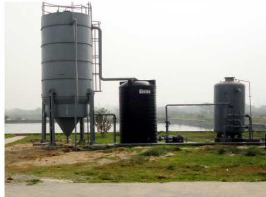
Continuous Sand Filter for Surface Water Treatment
