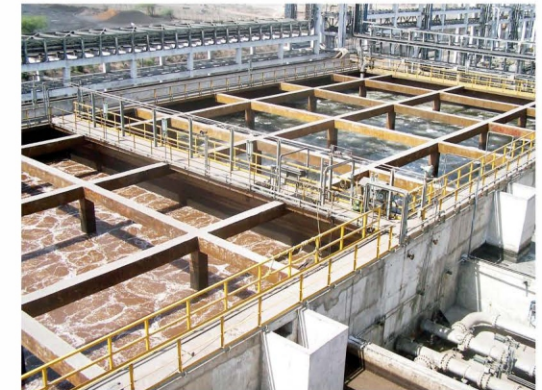
Effluent Treatment Plant at Refinery
