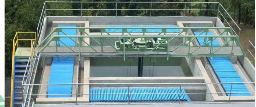
Ultra High Rate Clarifier for Textile Plant
