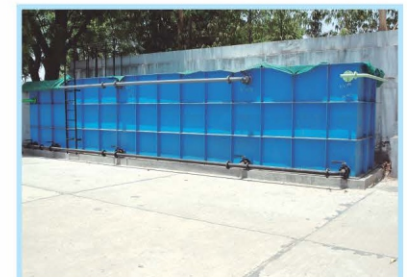
Fluidised Media Reactor at a Hotel
