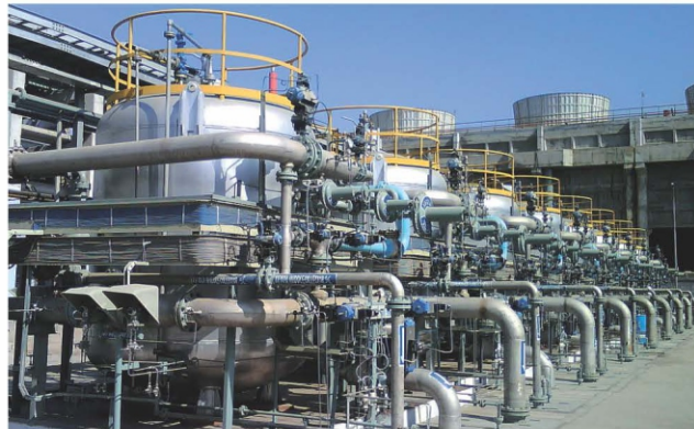
Demineralisation Plant at Petroleum Industry
