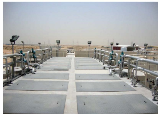
Membrane Bioreactor Plant at Industrial Area
