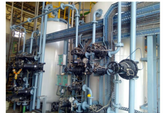
Glycol Purification for Chemical Plant
