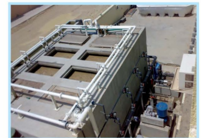
Membrane Bioreactor at Commercial Complex
